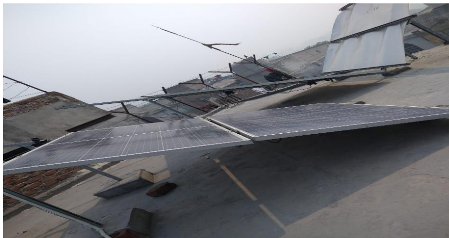
Figure 5: Aluminum sheet reflector with poly and mono crystalline PV modules
