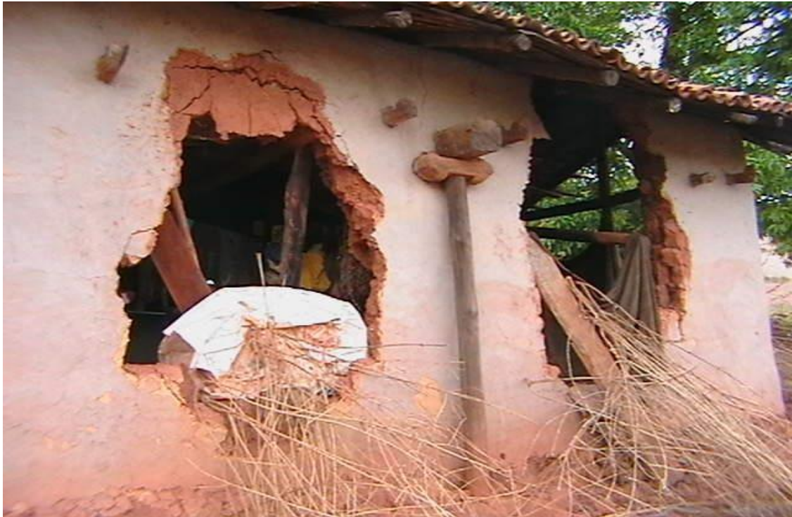
Plate –1. Shows house damaged caused by elephant.
