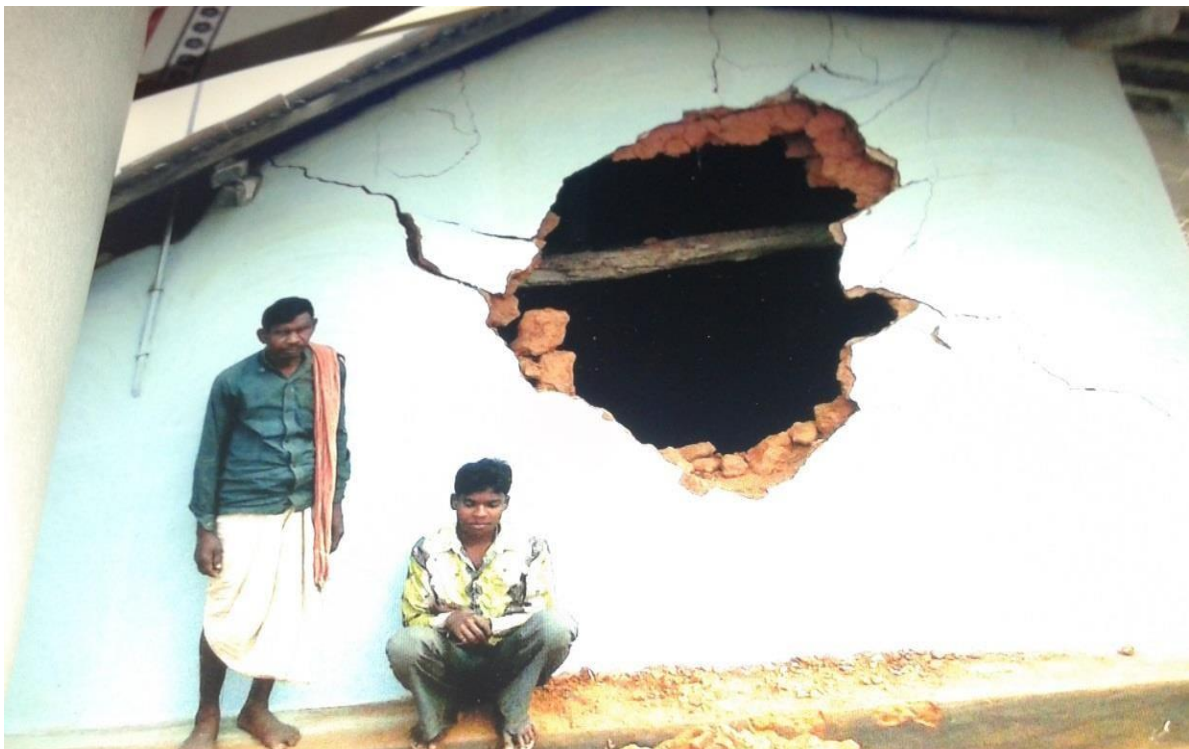
Plate – 4. Shows house damaged caused by elephant.
